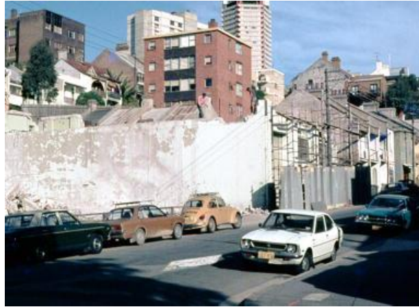
Figure 23: 118 McElhone Street, Woolloomooloo. Looking SE past the original site of the International Radio Coy on the left at 118 McElhone Street which is being demolished. Apartment block at the upper centre is the Oasis building at no 6 Windeyer Street. June 1979. Woolloomooloo photo collection: 62513, City of Sydney Archives.
